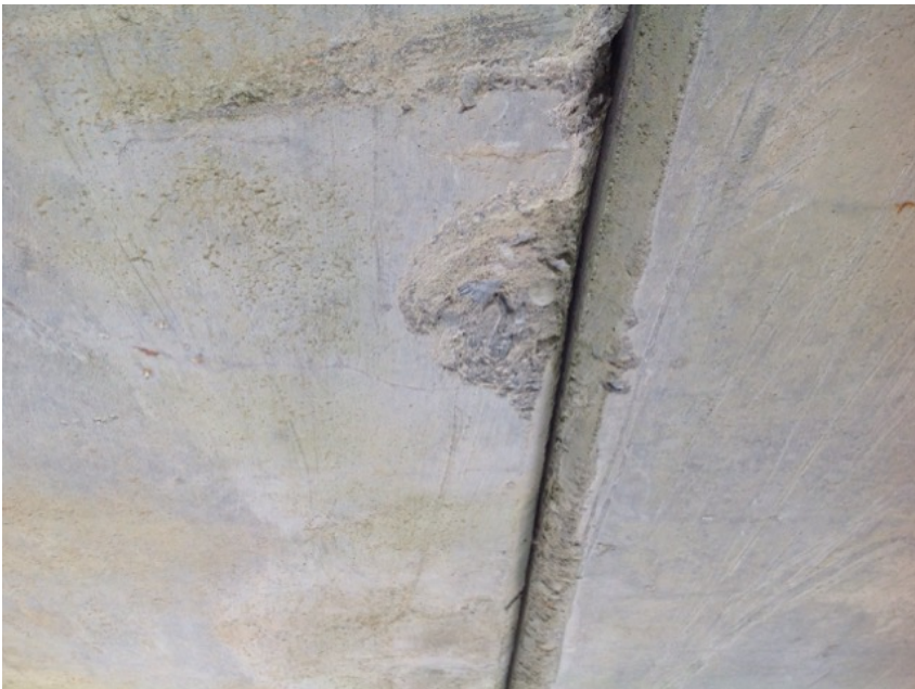
random concrete spall - noted throughout slabs but no rebar exposed
