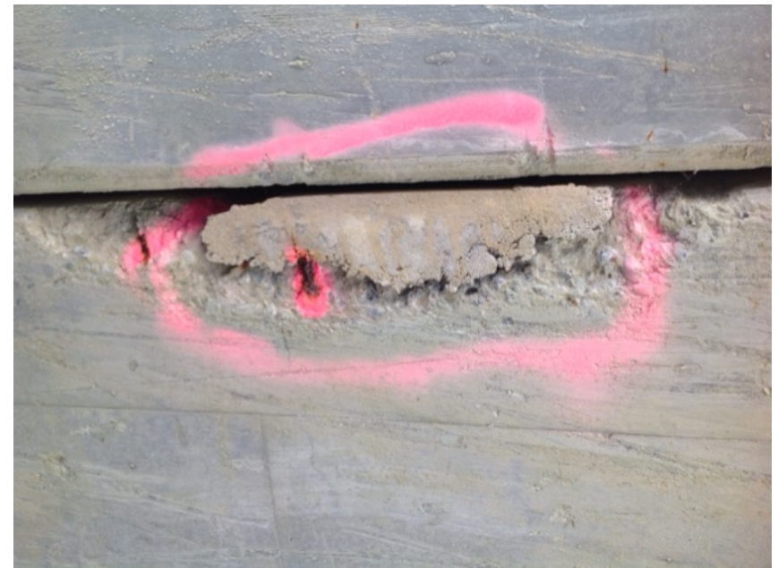
concrete spall with exposed rebar
