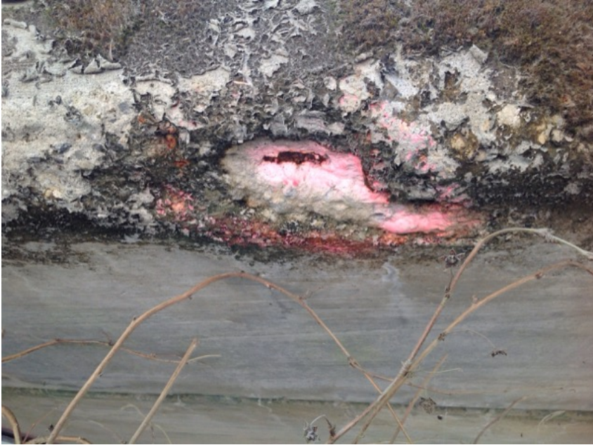
concrete spall with rebar exposed
